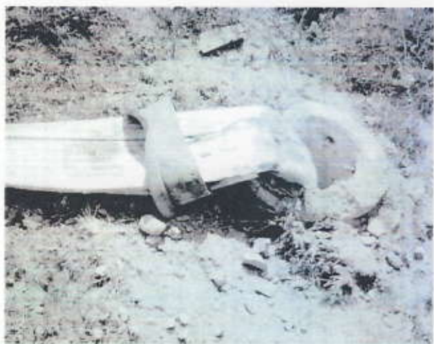
A KAPU® HE column that has sustained a collision along Highway 7 in Finland
